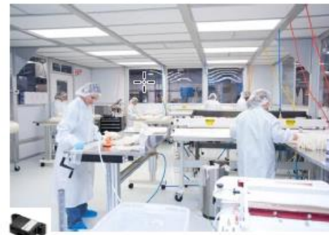
Clean room flow detection
