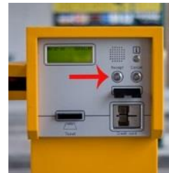
Parking Lot Ticket Dispensers
