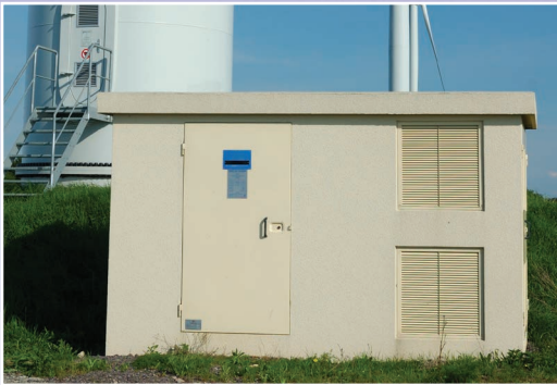
Substation and Control Room
