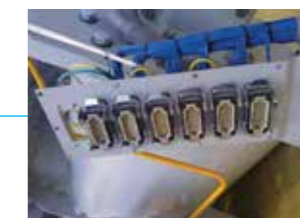
■ High-tension switch cabinet
